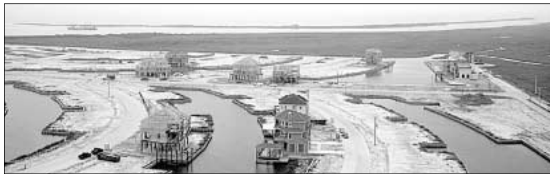
Construction continues throughout Harborwalk even as new sections are being opened to the public. Summerland was just released and has already sold. The 19 home sites on Saddlebunch will be released later in two weeks.
