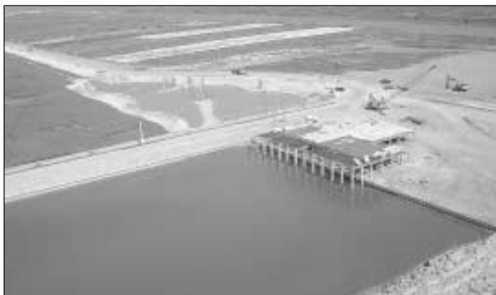
The coastal estuarine and inland marshes of the wetlands at Harborwalk provide nesting and wintering habitat for thousands of migratory birds and shorebirds. This photograph shows a bird's-eye view of the construction underway on Spoonbill's Restaurant and Bar.
